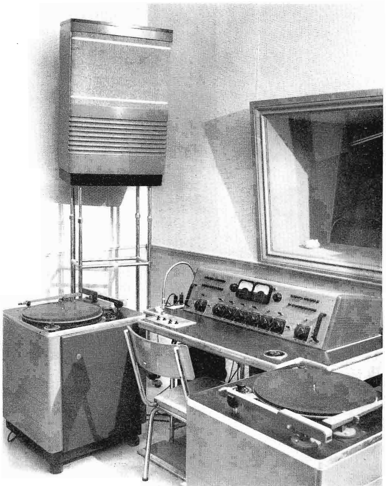
FIG. 18. Typical control studio. One of five similar control rooms. Note speaker's signal panel built into desk (left).
